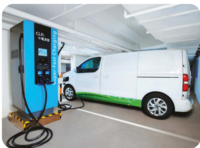
■ CLP's new network of EV charging stations in Hong Kong helps meet growing charging demand from commercial vehicle fleets.
