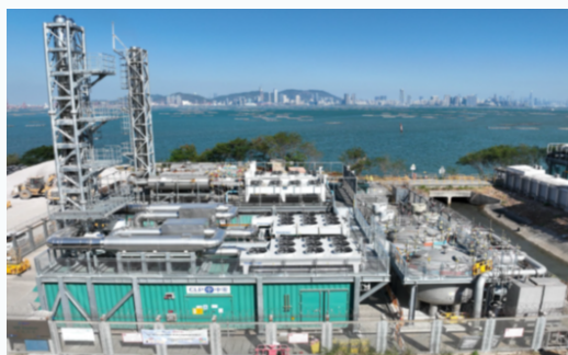
CLP Power's WE Station at the West New Territories (WENT) Landfill.
